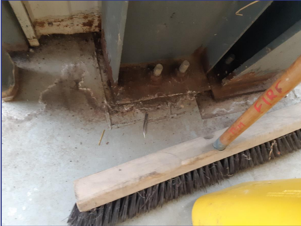
Photograph 5: View of corrosion to protection system of steel columns at ground level
