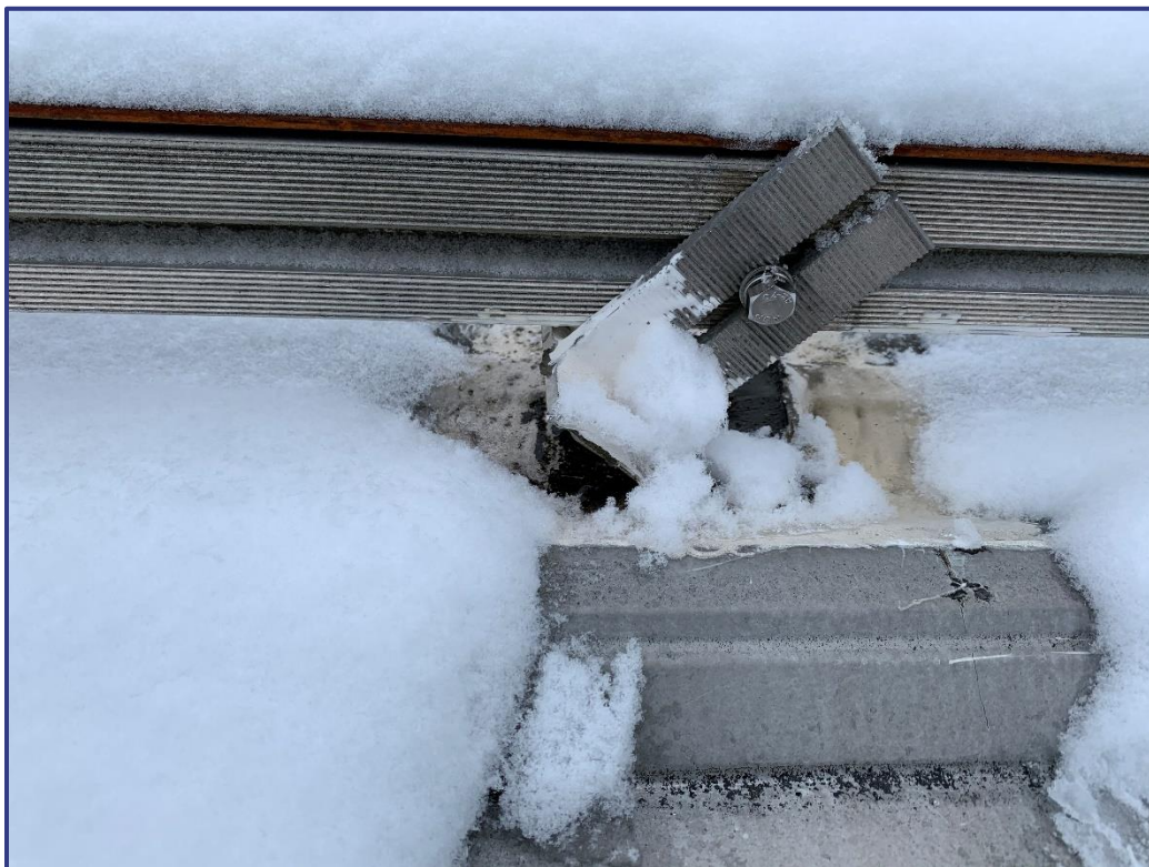
Photograph 8: Damaged caulking at bracket locations
