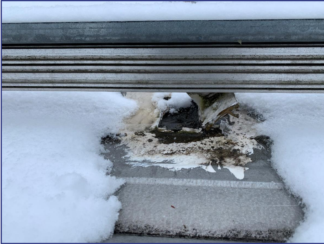
Photograph 7: View of solar panel brackets pulled away form roof
