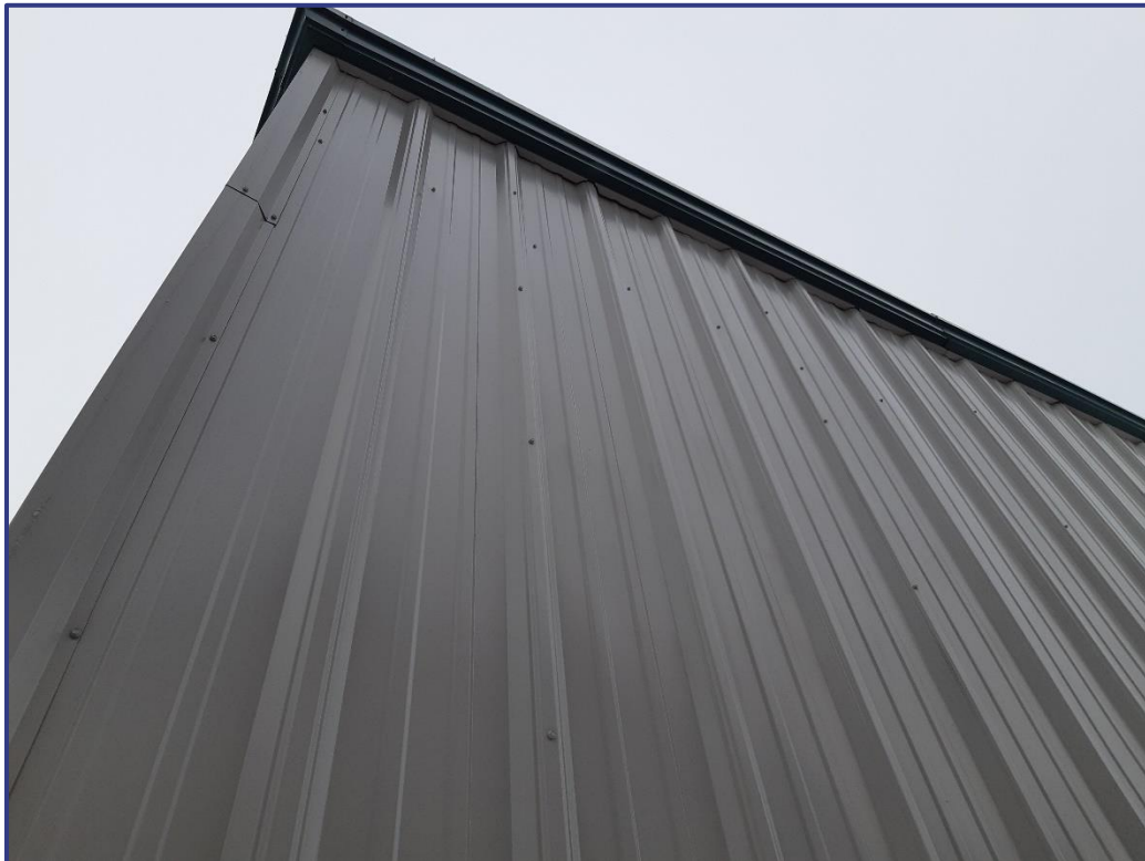
Photograph 12: View of no roof drainage
