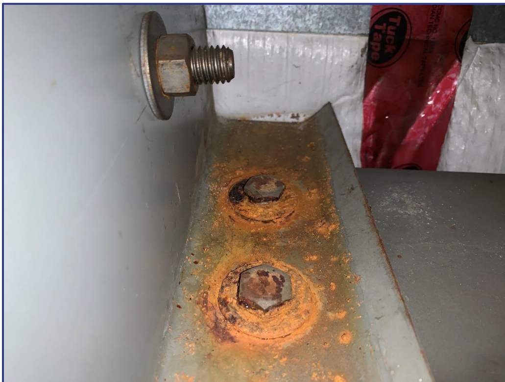
Photograph 6: Corrosion of bolts connecting purlins to steel frame
