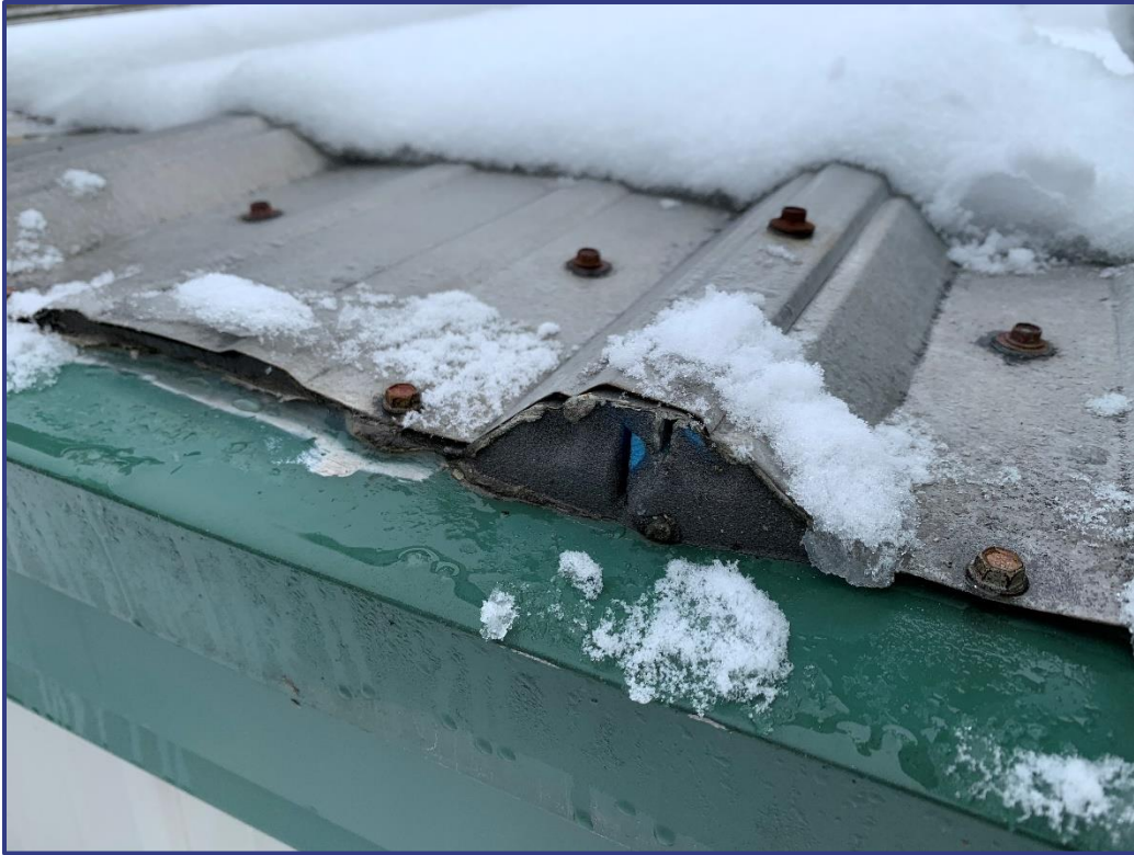
Photograph 9: Metal roofing cut back from edge of building flashing
