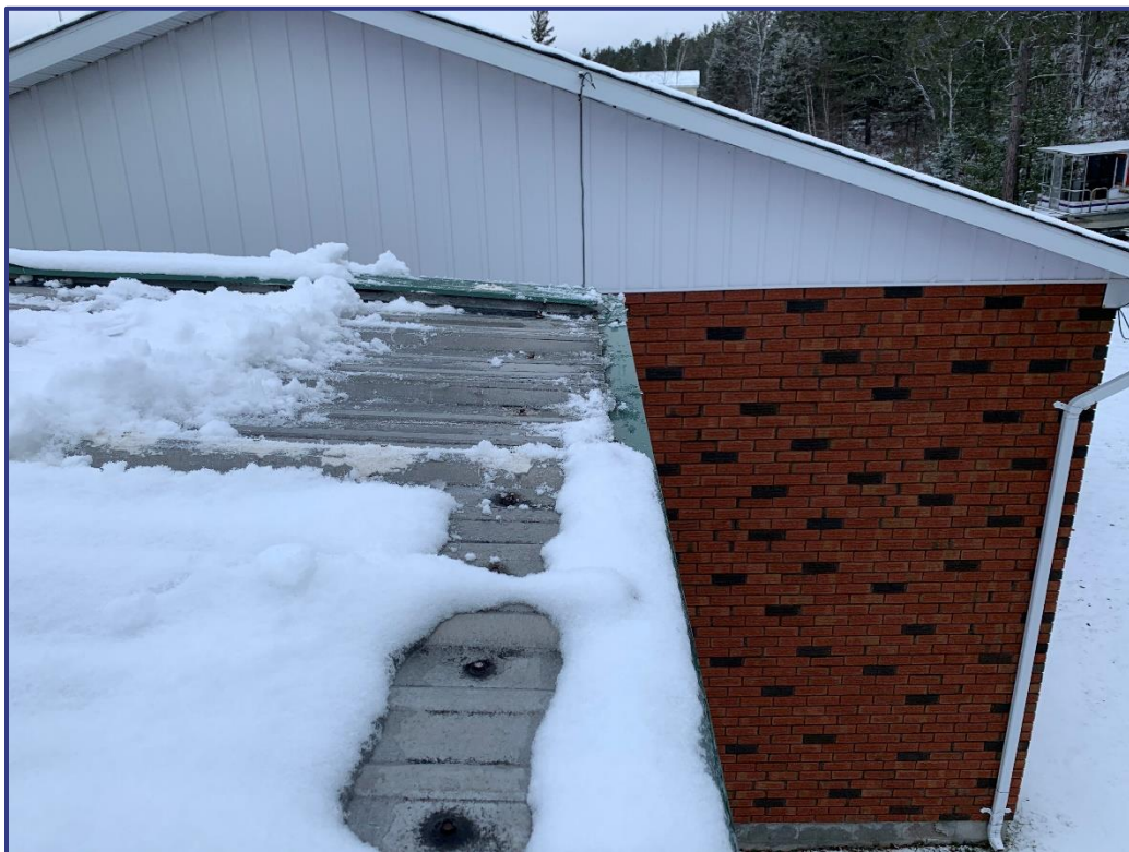
Photograph 10: Pooling water at low areas of roof edge
