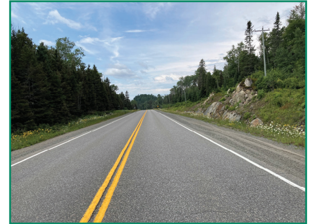
GWP 5033-22-00 (North): Highway 11 from 4.6 km north of Highway 64 northerly 11.4 km to 340 m south of Jumping Caribou Road
